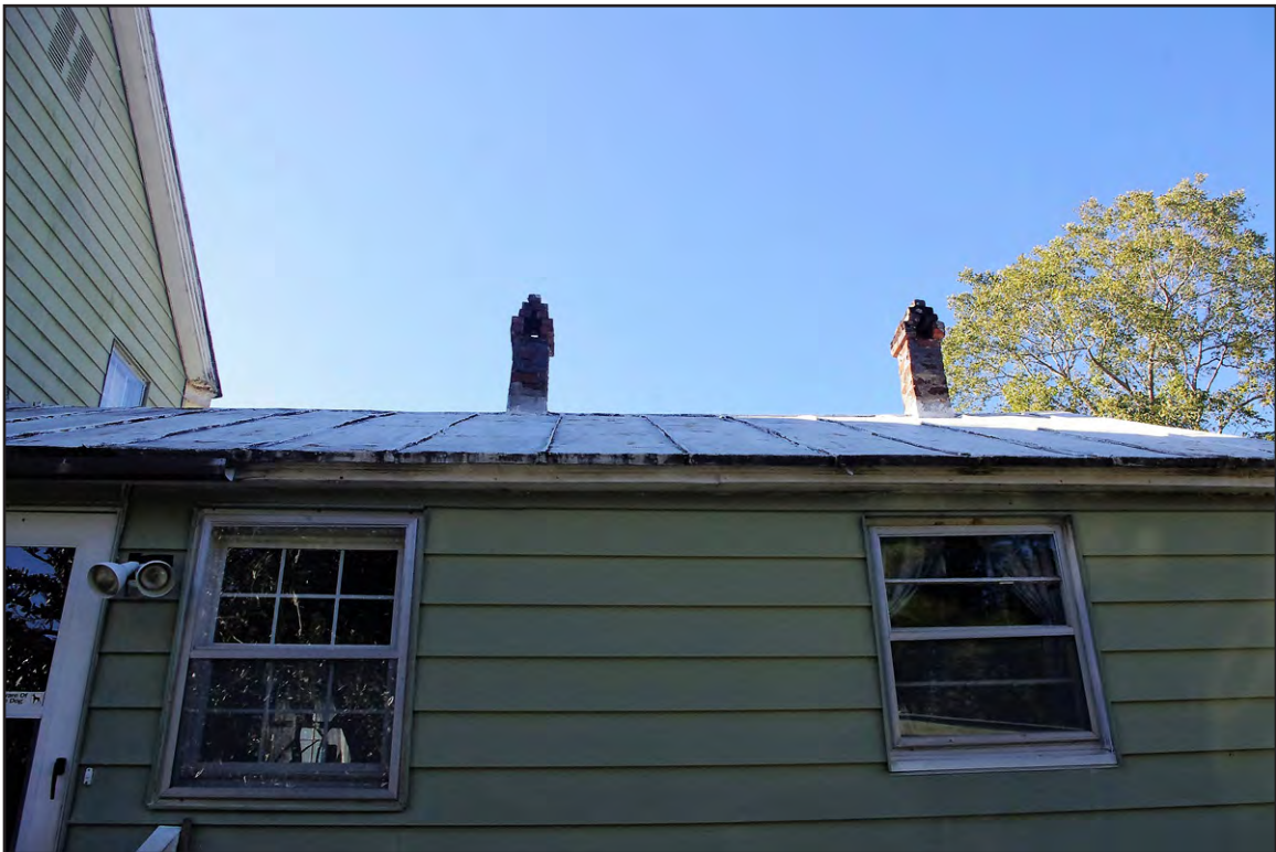
PLATE 35: Maggie E. Murdoch Watson House, East Elevation, Detail of Windows on Enclosed Rear Ell
