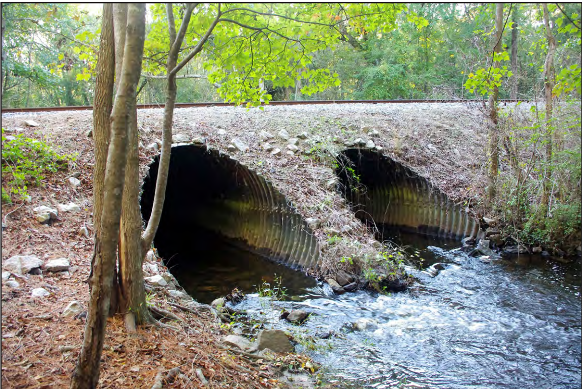
PLATE 51: Metal Culverts at Hull Swamp Creek Running Under Norfolk Southern Railway Line, Looking Southwest
